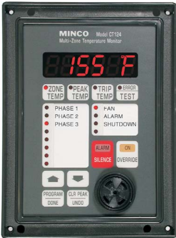
Zone Temperature (default display): Phase 3 of a transformer is reading 155°F. Relay 1, wired to cooling fans, has tripped.
