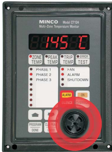
Alarm: The internal alarm has sounded and Relay 2 has tripped.
